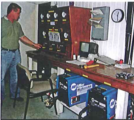
Miami Diver has found that the XMT 350 and XMT 456 multi-process inverters from Miller Electric Mfg. Co. provide portability and consistent weld quality.
